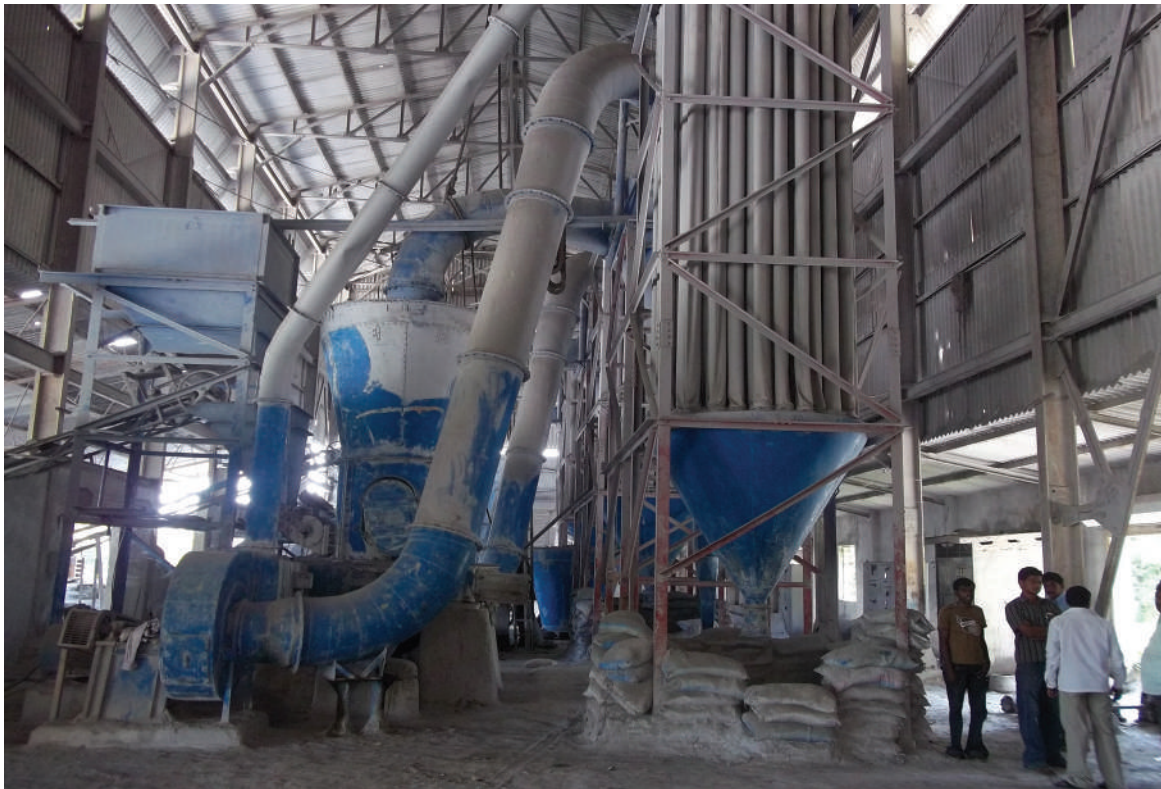
Fig 6.12: Crushing and packing plant
